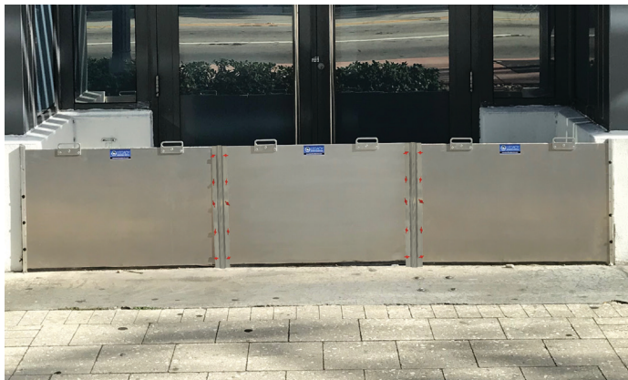
#5129MA mounted to front of hotel entrance.
