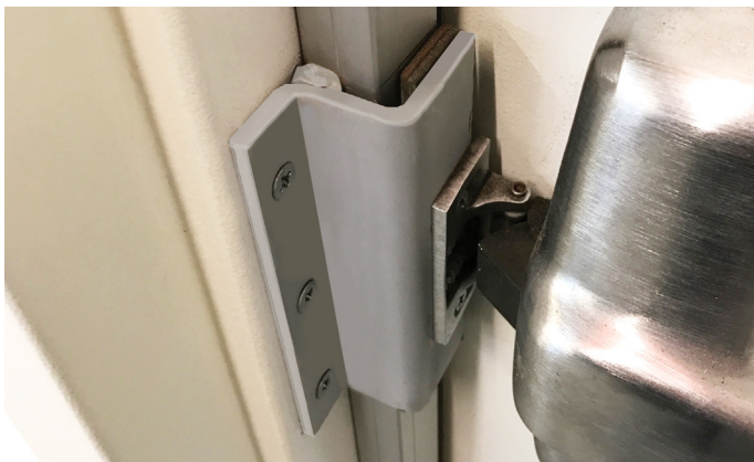
#5078SPB installed at the door strike.
