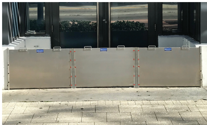
#5129MA mounted to front of hotel entrance.
