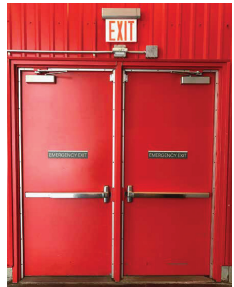
#5077 installed in conjunction with #5077SPB.
