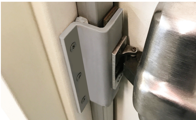
#5077SPB installed at the door strike.
